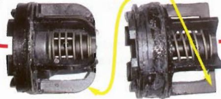
007-M3 'cage' modules are different for check valves 1 and 2.
